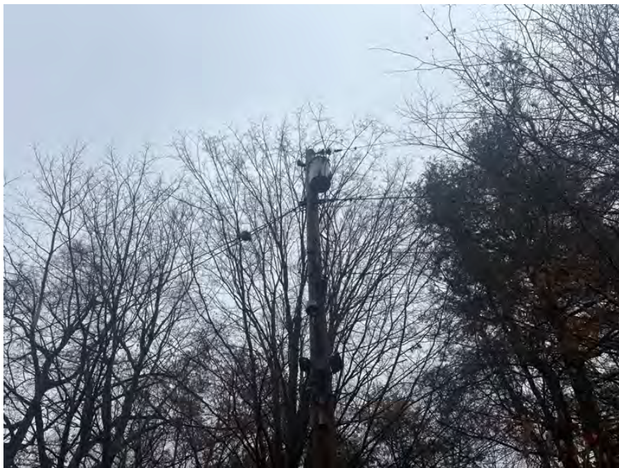
Photo 10 : Representative view of pole-mounted transformer on the center of the Subject Property, along the northern portion of Camp Sunset Road. No staining or leaks were observed.
