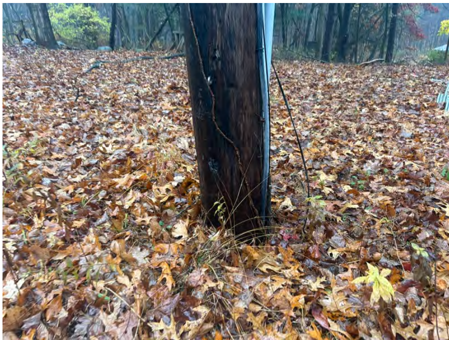
Photo 12 : Representative view of pole-mounted transformer on the center of the Subject Property, along the northern portion of Camp Sunset Road. No staining or leaks were observed.
