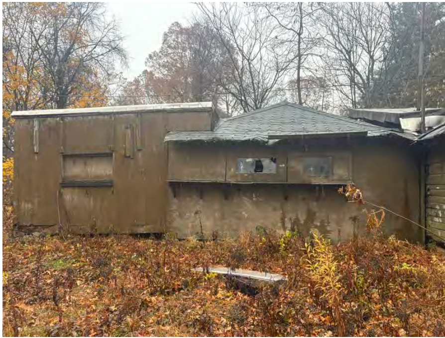
Photo 15 : View of dilapidated structure
